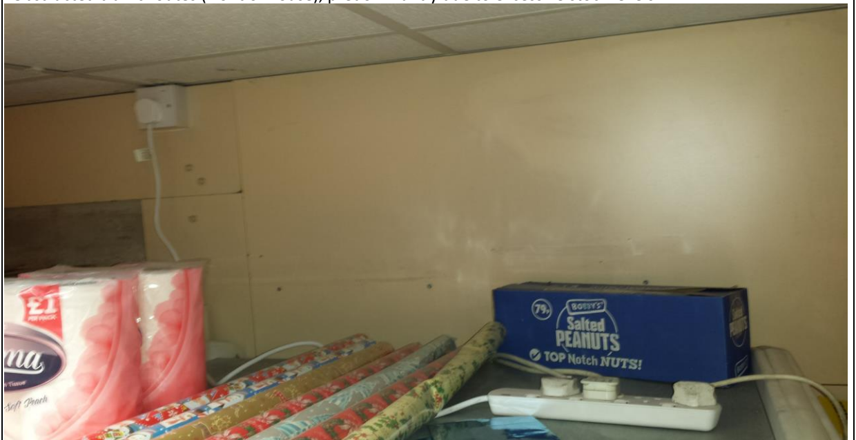
Picture showing 1 socket feeding 3 drinks fridges - under resourced in regards to electrical sockets. Overloaded electricity is a major cause of fire and this extension lead is next items that would easily combust if the socket or wires overheated.
